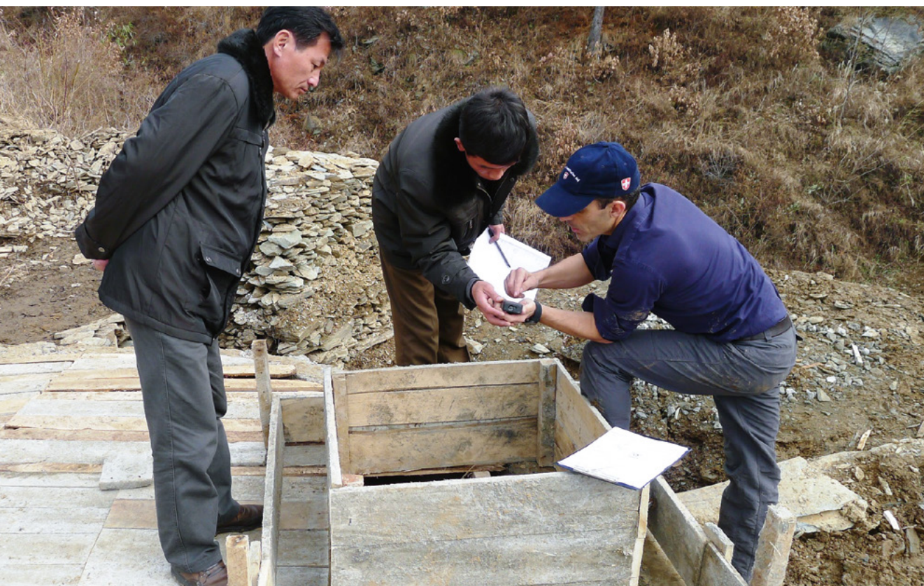
Construction of a water reservoir. The source protection perimeter will be fenced afterwards. Democratic People's Republic of Korea. © Guillot, 2013, SHA
