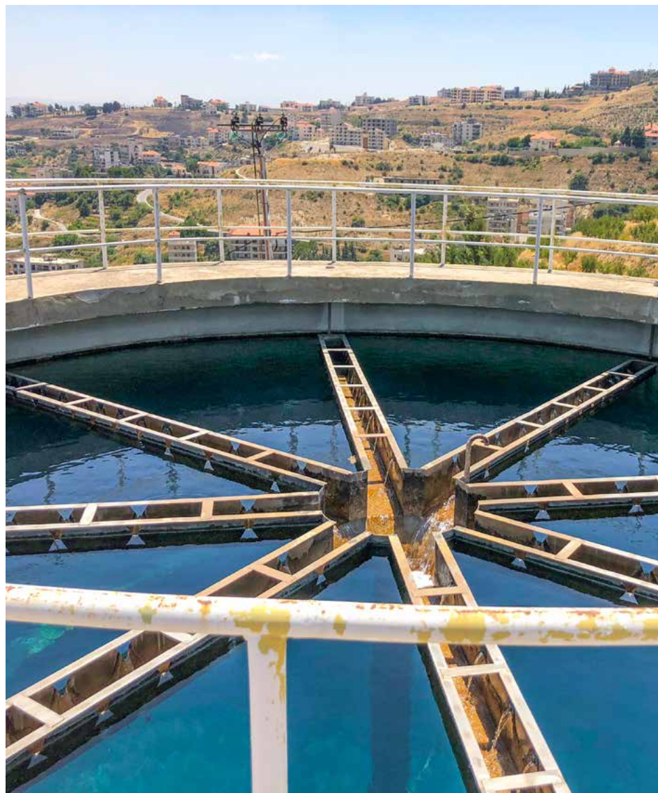
Job Janin water treatment plant in Bekaa Valley, Lebanon, supported by SDC. © Embassy of Switzerland in Lebanon
