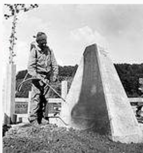
Construction of anti-tank obstacles in the 1940s. They were also nicknamed "Toblerone" due to their resemblance to the famous Swiss chocolate bar. © Theo Frey/Swiss Federal Archive Bern
